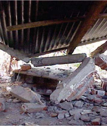
A childcare center destroyed by the 2001 earthquake.
